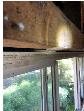
Photograph 22: Flat cement sheet fragments packers used between window frames and timber/brick framework (Asbestos detected in packer fragments)
