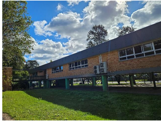
Photograph 14: Building B00F external area (Asbestos detected in window putty)
