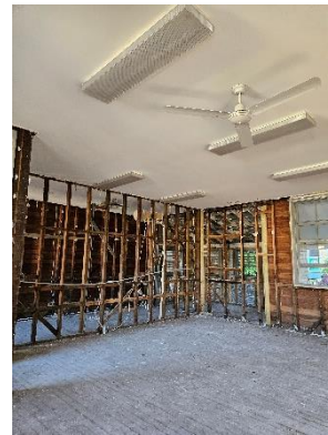
Photograph 10: B00C internal areas (Asbestos fibres detected in dust on floor)
