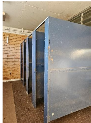
Photograph 18: Toilet cubicles in building B00B ground floor toilets (Asbestos detected in compressed cement sheet cubicle wall linings)
