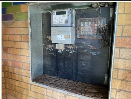
Photograph 23: Electrical distribution board ground floor B00F (Asbestos detected)
