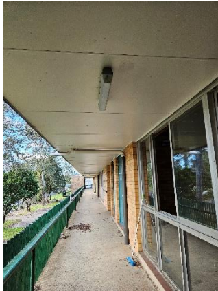
Photograph 15: Building B00F walkway/movement area (Asbestos detected in flat cement sheet ceiling lining)
