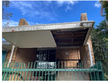
Photograph 20: Damaged ceiling lining to B00F stairway/movement area (Asbestos detected in flat cement sheet ceiling lining)
