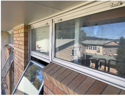
Photograph 19: External windows B00A (Asbestos detected in window putty within the rectangular top windows)
