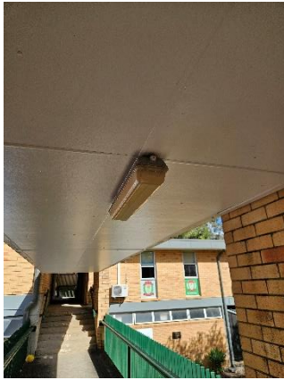
Photograph 13: Movement area between building B00B and B00F (Asbestos detected in flat cement sheet ceiling lining)
