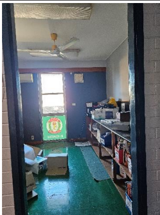
Photograph 11: Building B00B photocopy room (Asbestos detected in green floor tiles)
